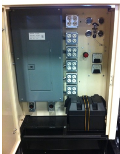
Customized AC electrical distribution panel
