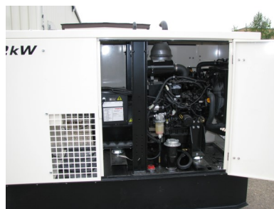
Large service access doors
