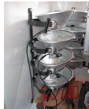
Light storage bracket (installed in building)
